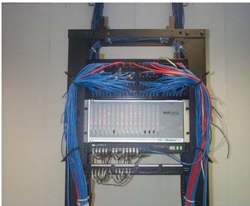
After the Move: Untangled and Re-Wired
